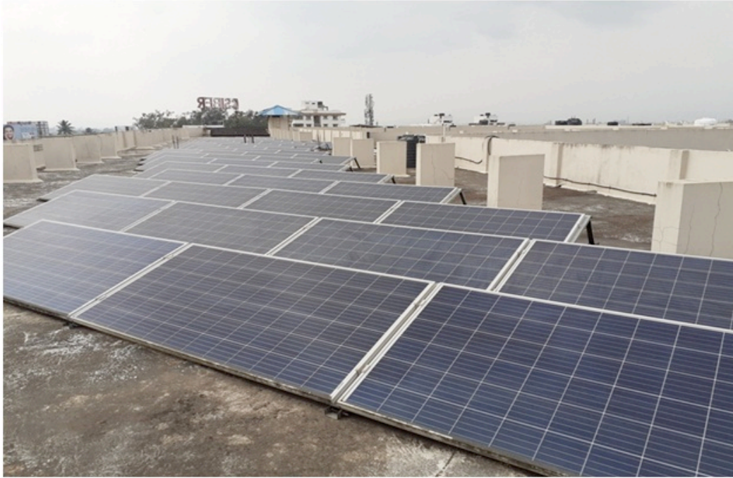
Solar power generation PVC panels on Roof top of the institute
