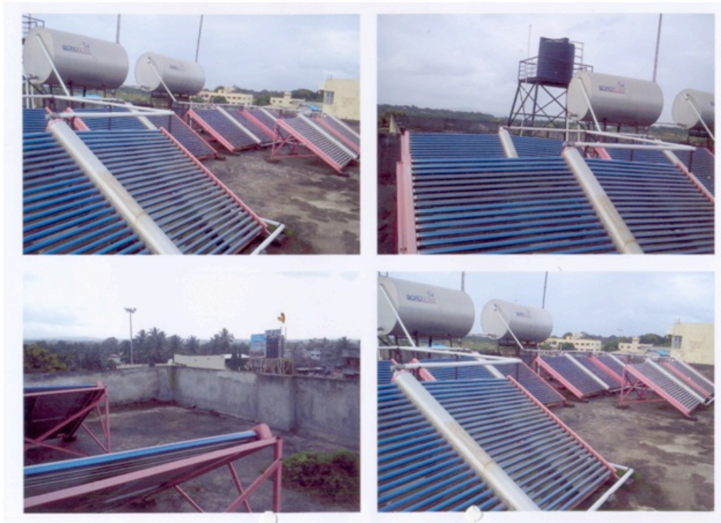
Solar Water Heaters at Boys Hostel
